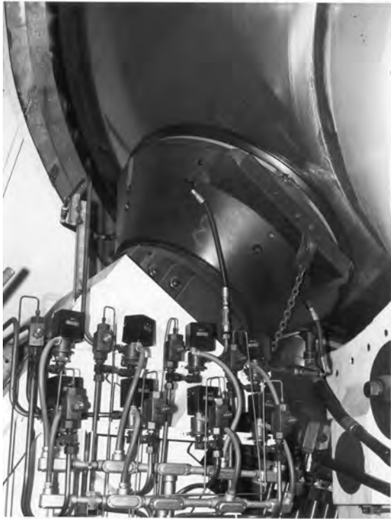
The spherical bearing sitting atop one of the hydraulic support pads.
