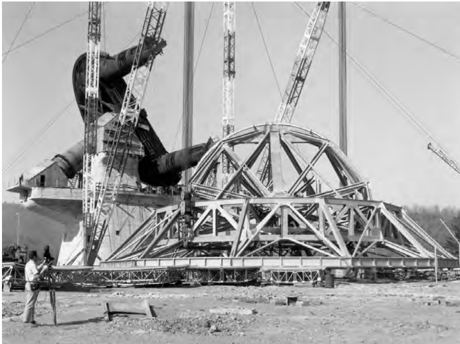
Top: The backup structure nearing completion on the ground in 1963. Bottom: Preparations for the lift into place on the yoke in November 1964. Film-maker Peter B. Good documents the procedure.
