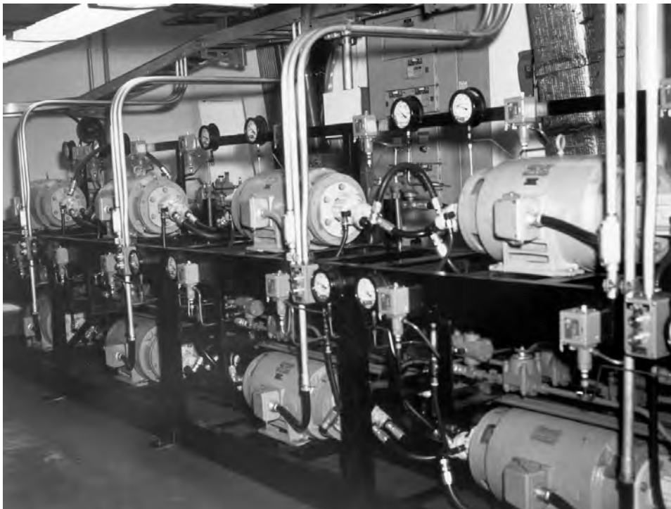
Some of the hydraulic pumps which supply oil to the bearing.
