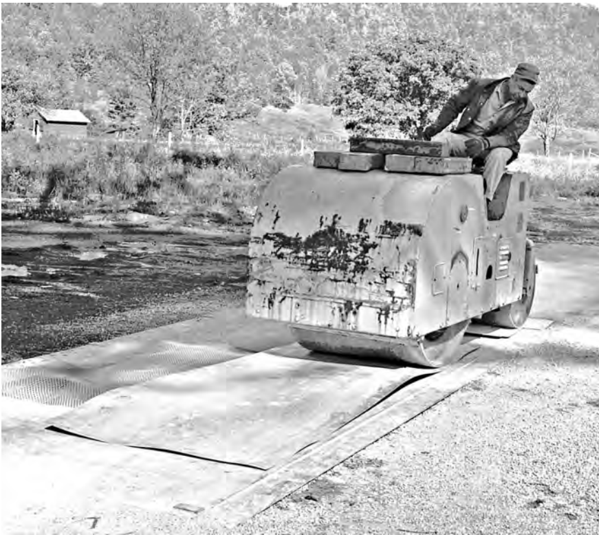
Top: The original surface showing its poor condition in September 1966. Bottom: Rolling over the original surface in an attempt to flatten it, October 1966. Fred Cole is operating the roller.
