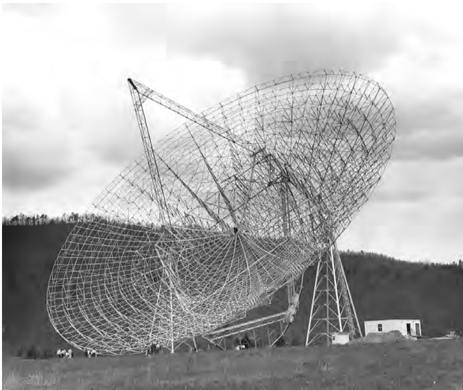
Top: Construction of the box girder, October 5, 1961. Workers are inspecting one of the gusset plates.
