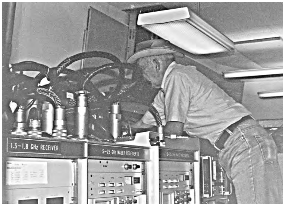
Carl Chestnut working on the receiver back ends in the 140 Foot control building, August 1990. [photo courtesy G. Liptak]
