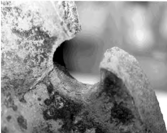
A bolt hole along the fracture line of the gusset plate.
