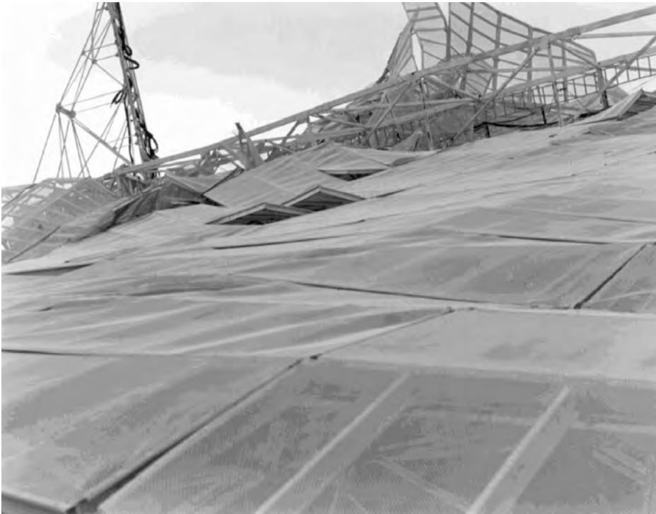
View from the north of the surface with the feed legs and traveling feed at left. The traveling feed penetrated the ceiling of the control building.
